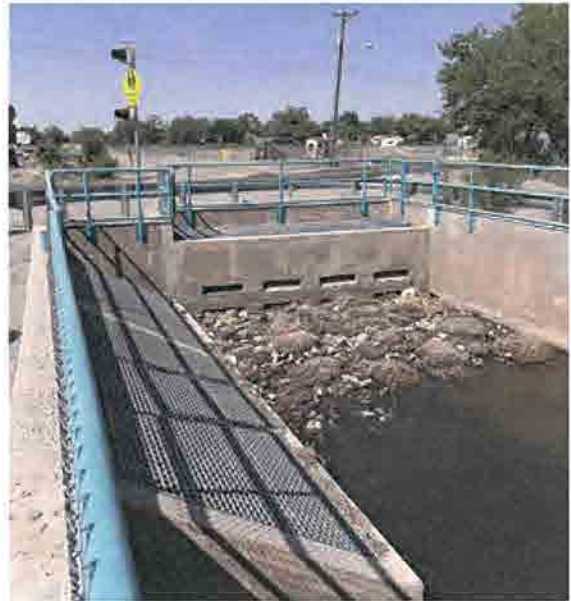
FIGURE 17. WATER FILTRATION AT ARENAL RD. CROSSING
