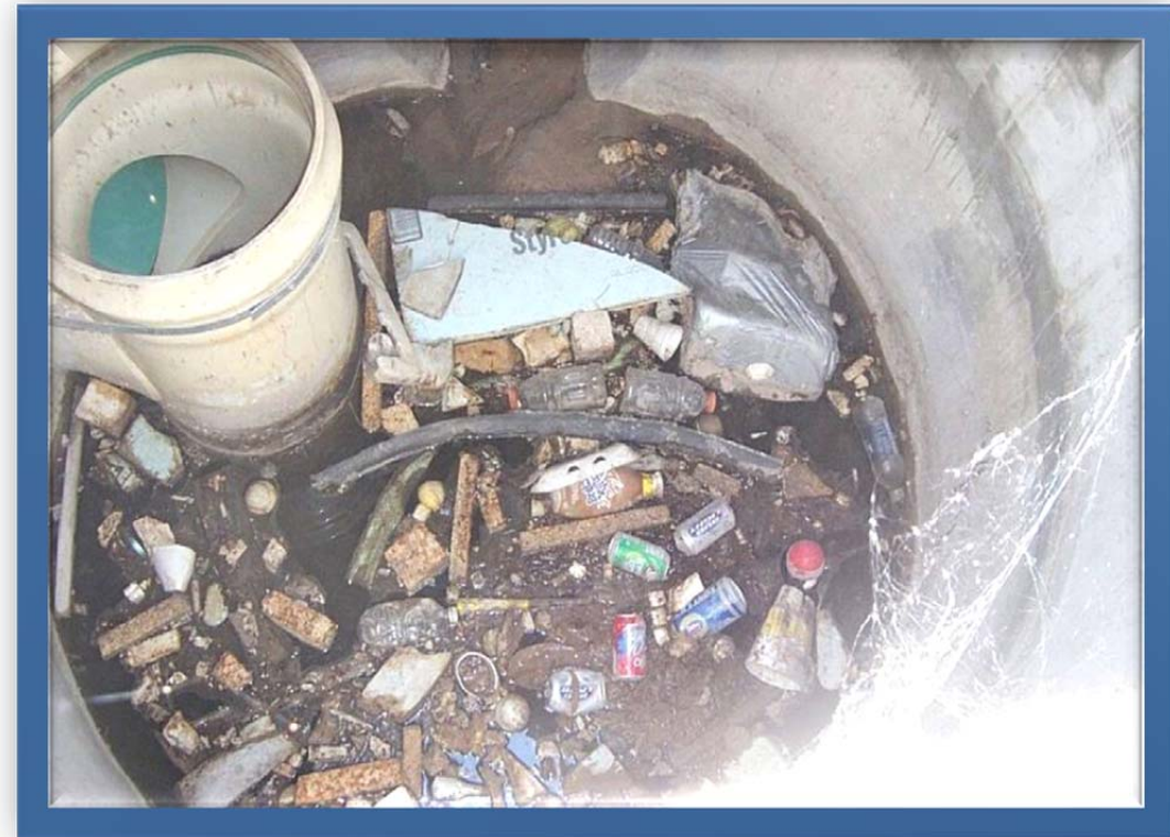
Water Quality Manhole (Source: Bohannon Huston, Inc.)
