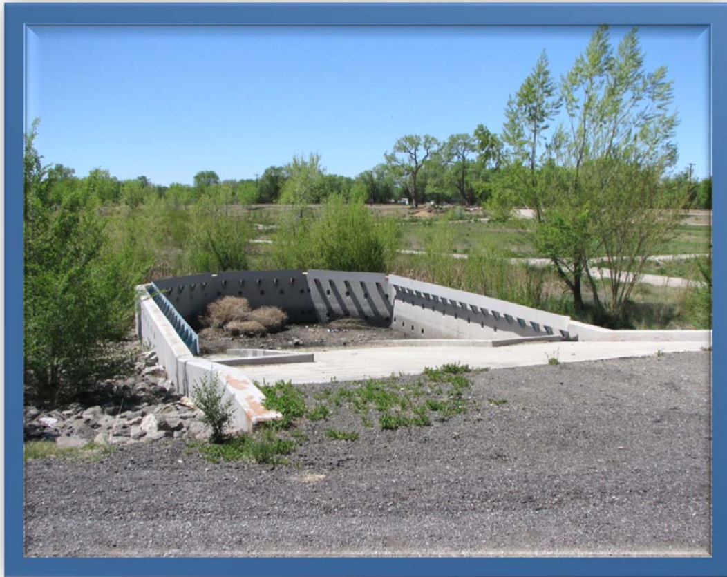
Sanchez Pond Debris Removal Structure (Source: Bohannon Huston, Inc.)
