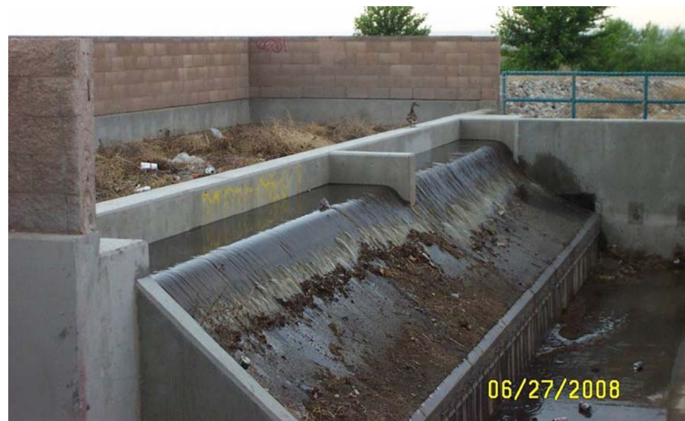
Coanda Screen on North Pino Arroyo. AMAFCA Water Quality BMP.
