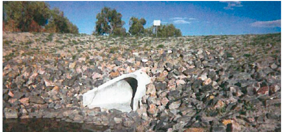
FIGURE 6.10.28 Unprotected Culvert Outlets Cause Downstream Erosion
